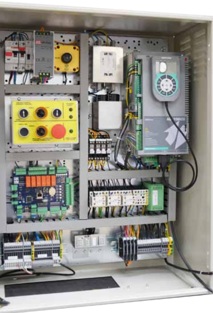
Eagle control panel for lifts
